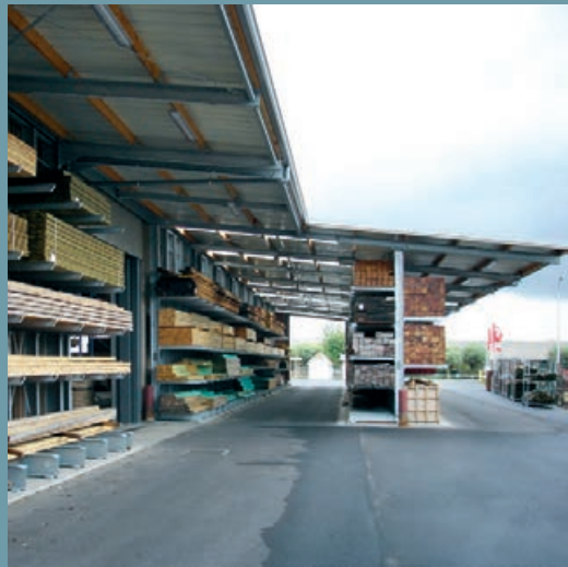
Fully enclosed rack-clad warehouse with additional open annex of a covered, double-sided cantilever-racking row. Incl. lighting and clear panels over the aisles.
