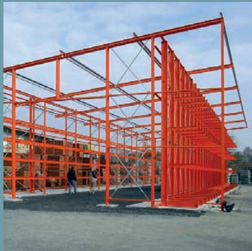
Rack structure, consisting of cantilever and pallet racks. Substructure including gable wall, shortly before the panelling. Block and sleeve foundations structurally computed.
